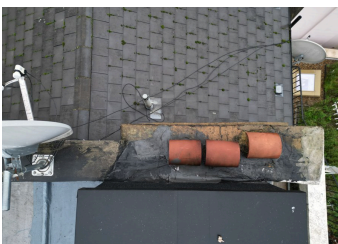
Close range · patched parapet coping and moss on slates
