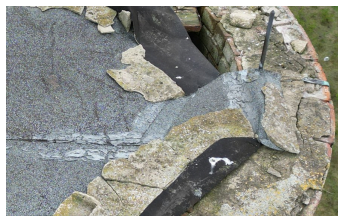
Capping · displaced copings and torn cap covering
