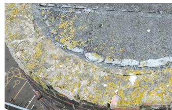
Close range · lichen, open joints and loose units
